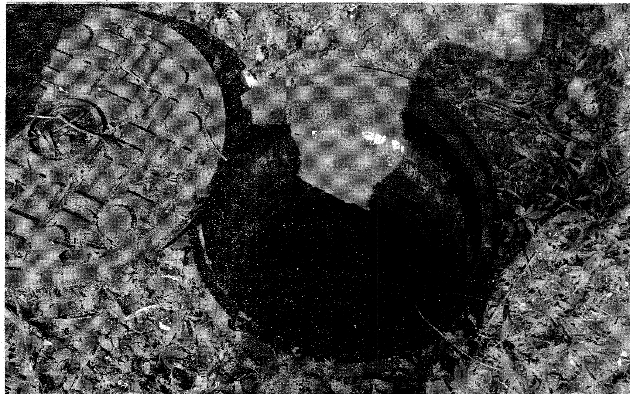
1 D-3 INFLUENT MANHOLE NO. 49-1070
