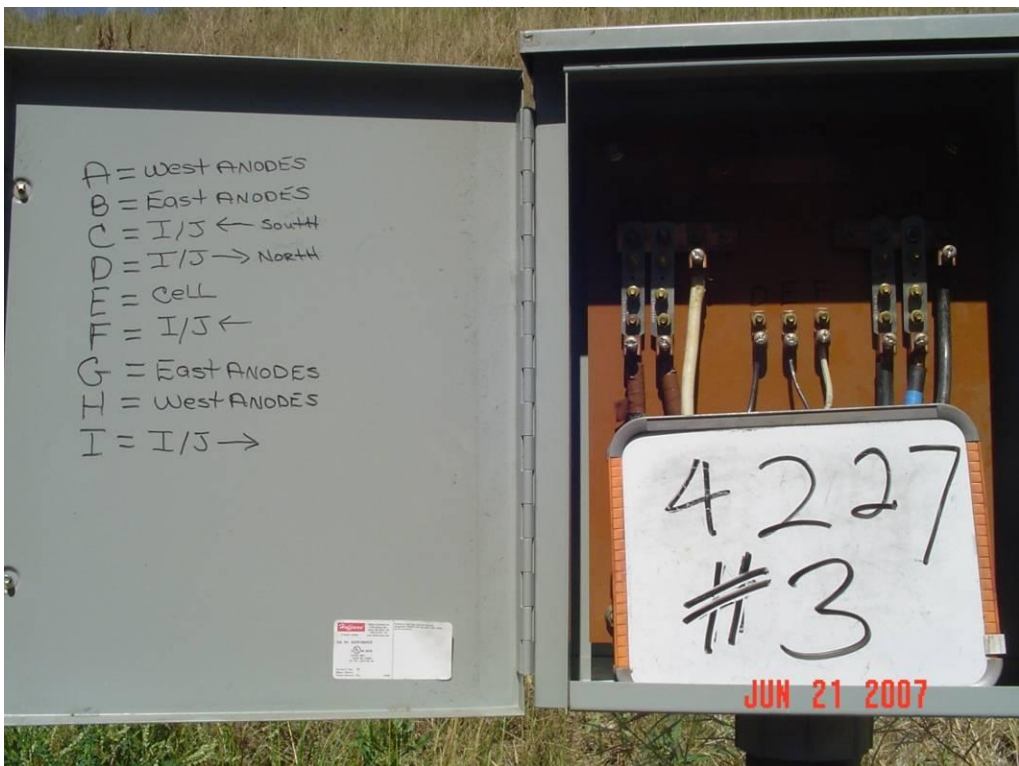
Figure 235 - Test Station 4227-3 close-up
