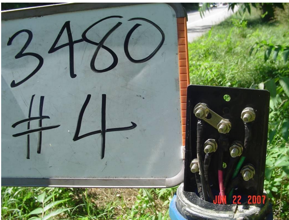
Figure 212 - Test Station 3480-4 close-up
