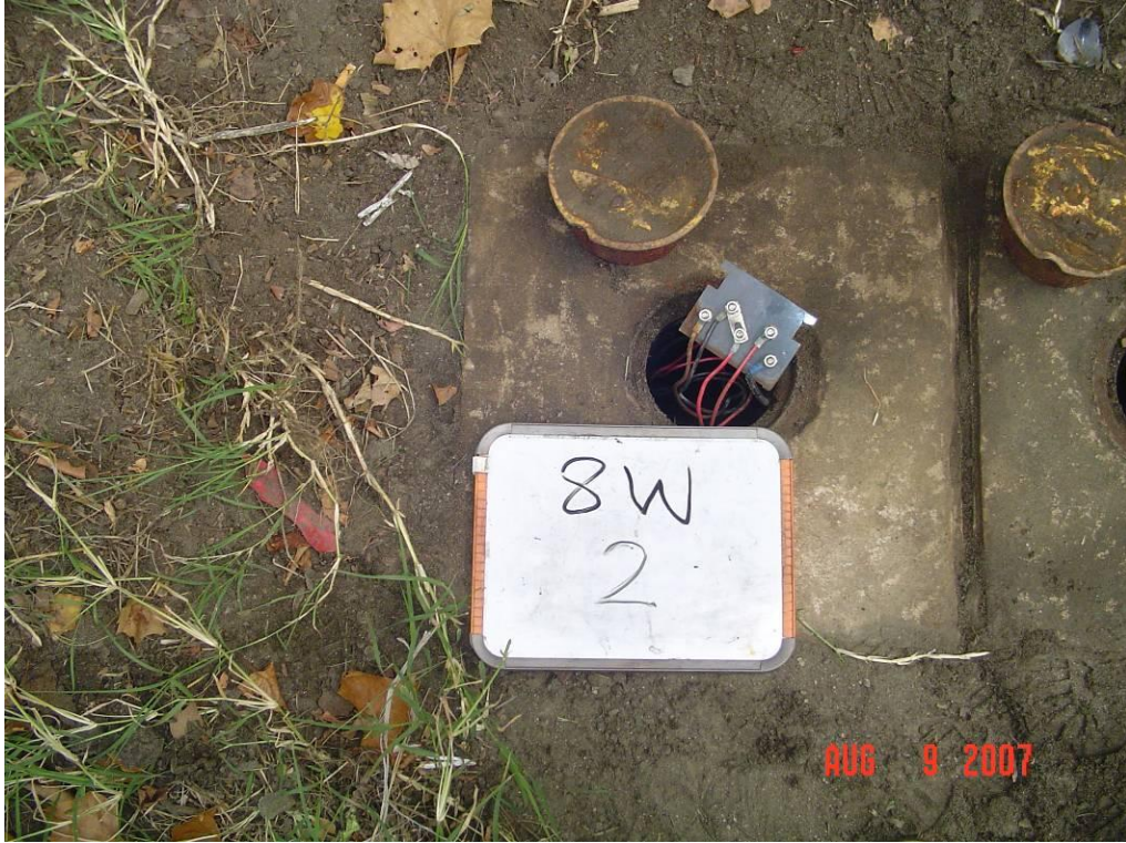
Figure 59 - Test Station 8W-2 close-up
