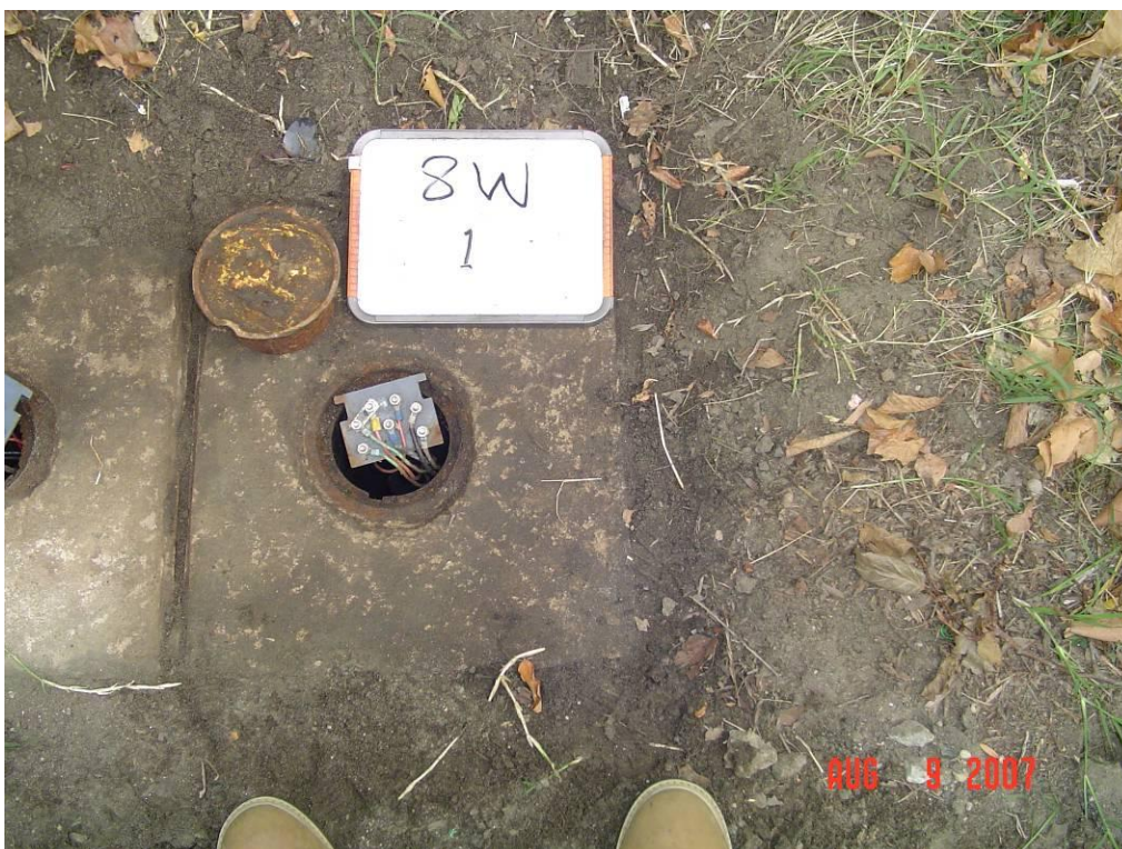
Figure 58 - Test Station 8W-1 close-up
