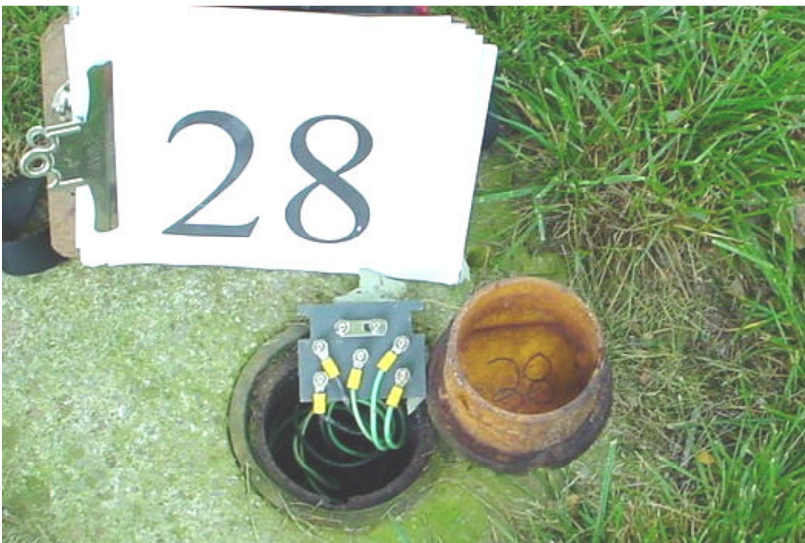
Figure 55 - Test Station #28, close-up
