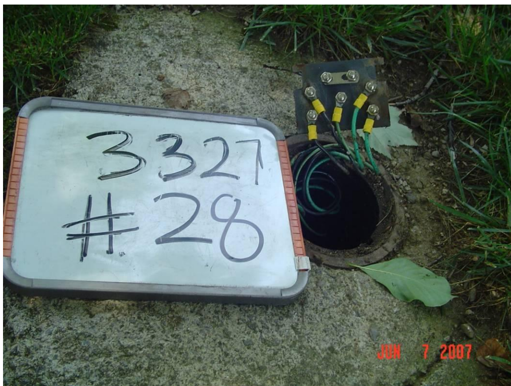
Figure 168 – Test Station 28 close up
