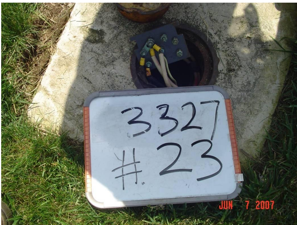
Figure 158 – Test Station 23 close up
