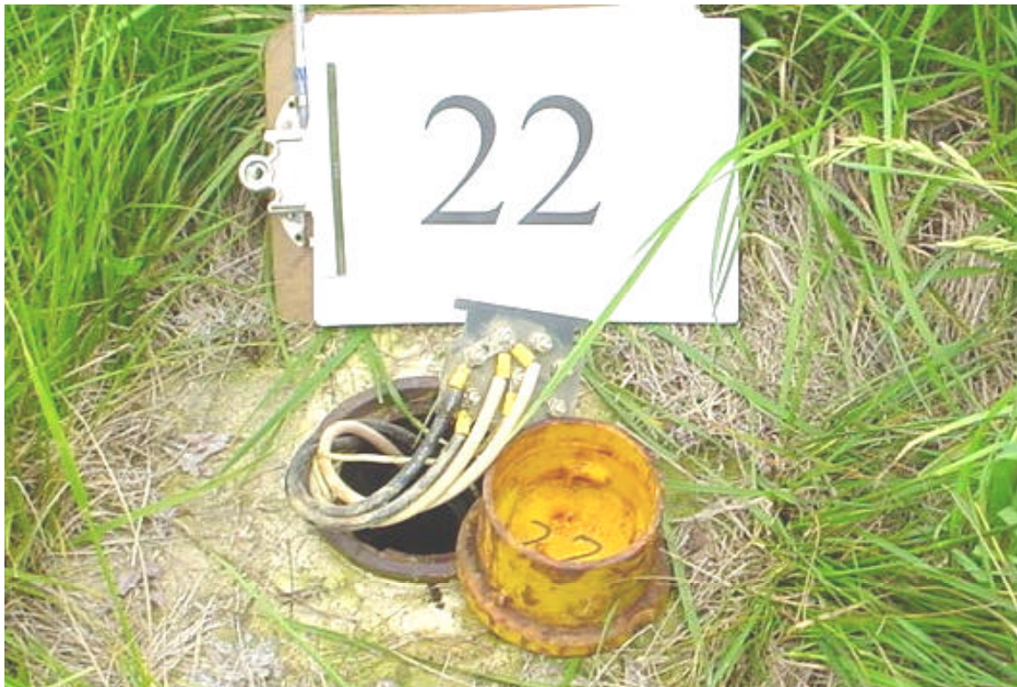
Figure 43 - Test Station #22, close-up
