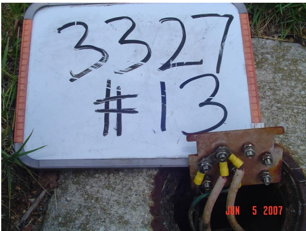
Figure 146 – Test Station 13 close up
