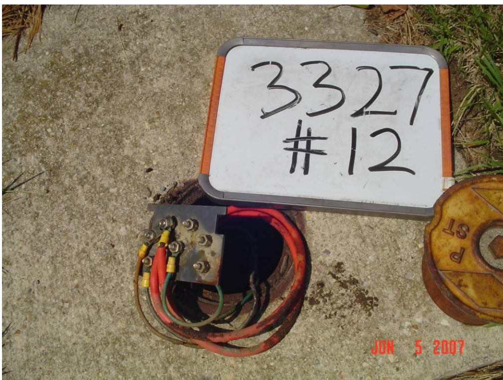
Figure 144 – Test Station 12 close up
