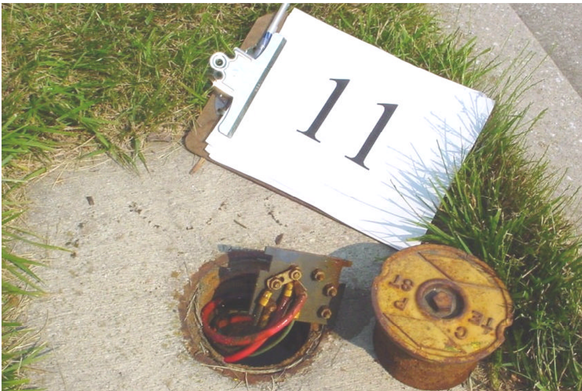
Figure 29 - Test Station #11, close-up
