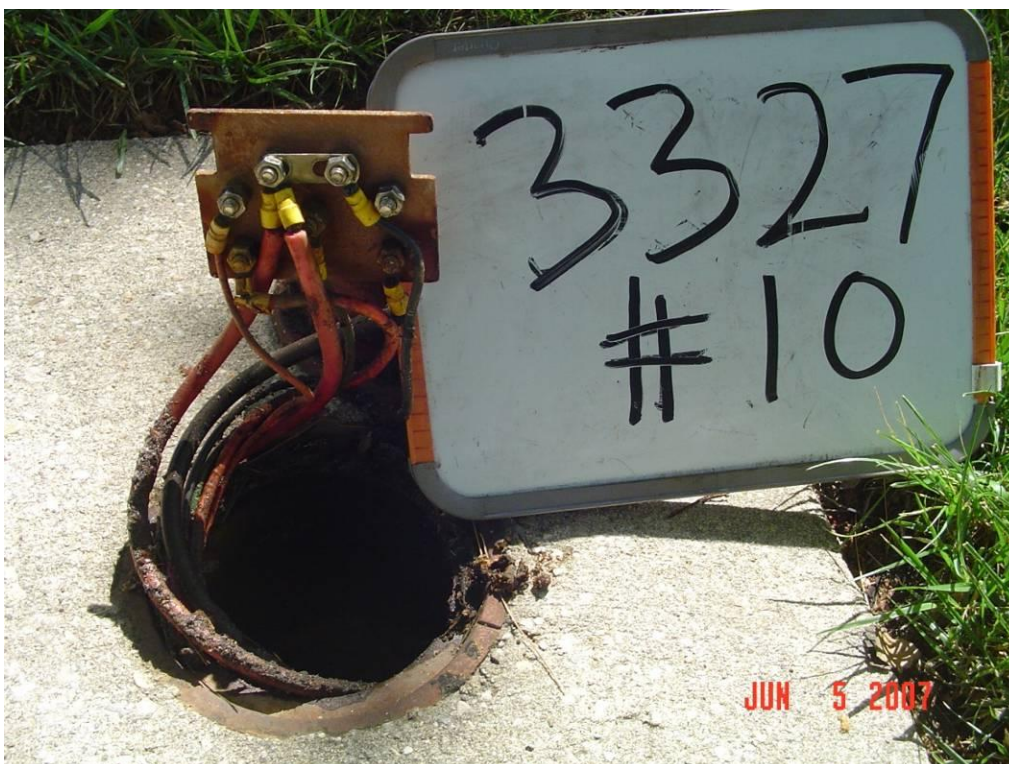
Figure 140 – Test Station 10 close up
