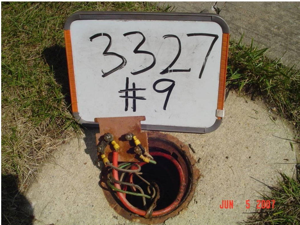
Figure 138 – Test Station 9 close up
