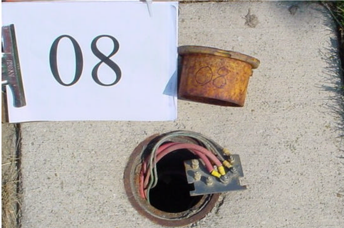
Figure 23 - Test Station #8, close-up
