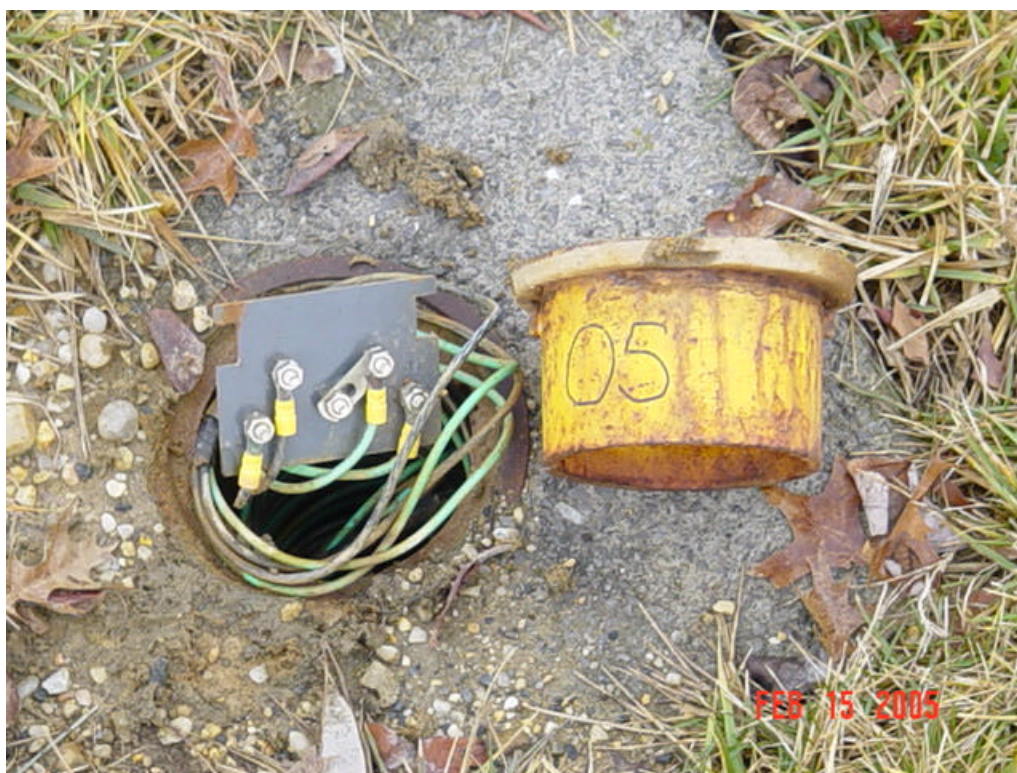
Figure 136 – Test Station 5 close up
