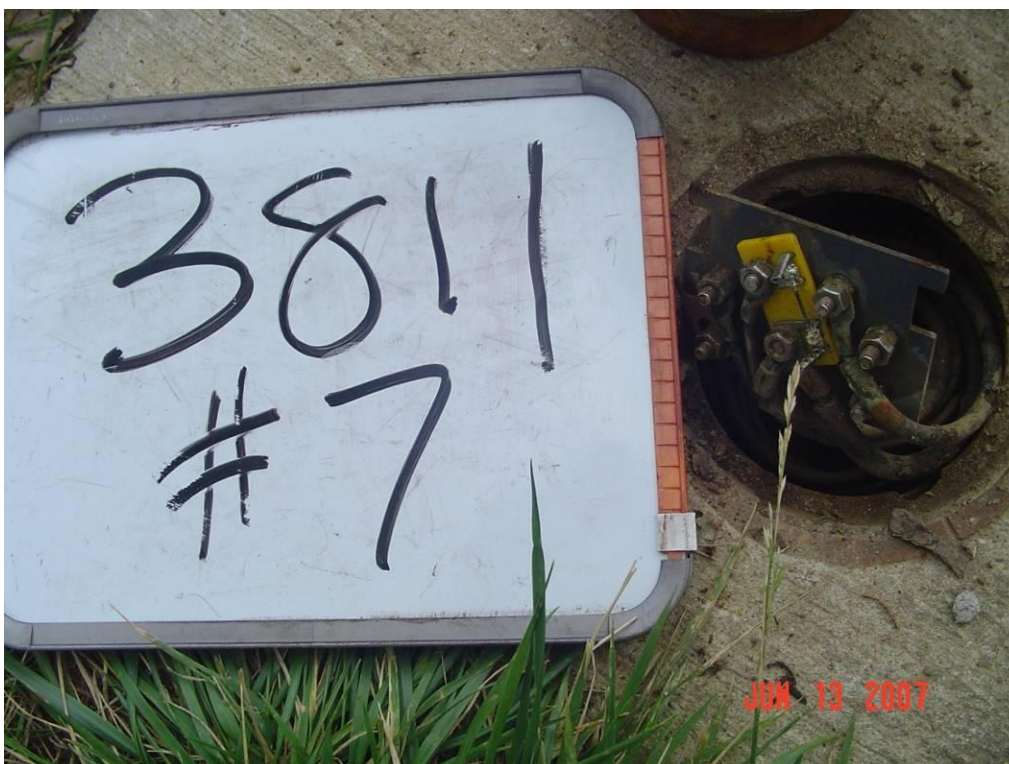
Figure 197 - Test Station 3811-7 close-up
