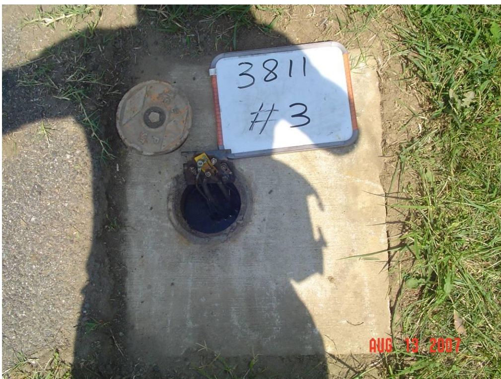
Figure 190 - Test Station 3811-3 close-up
