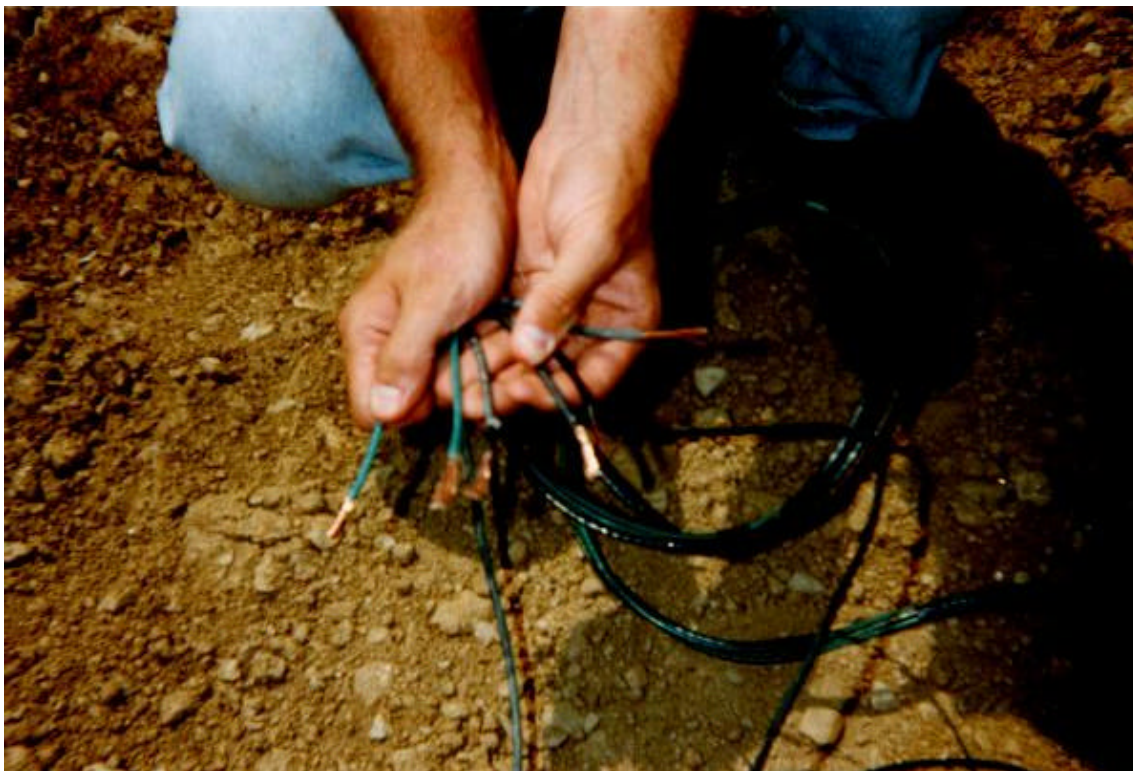
Photo 18. Test Station South of MD 108 Overpass - Test Wires
