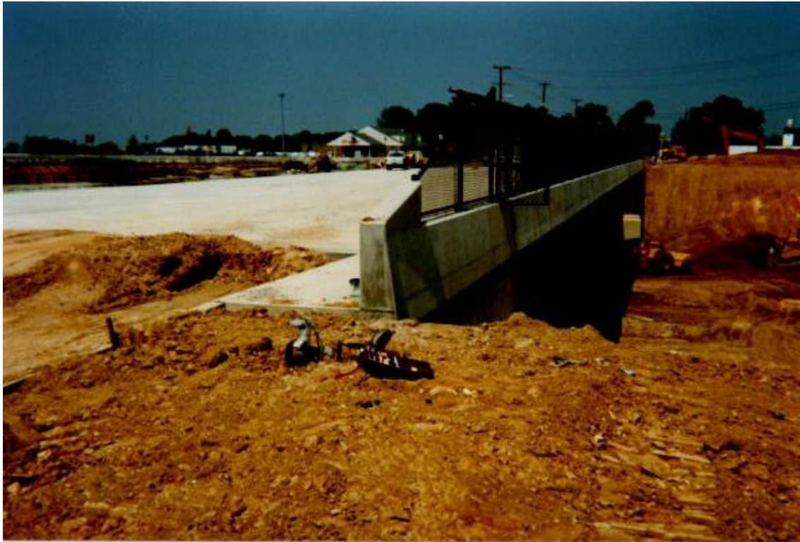
Photo 17. Test Station South of MD 108 Overpass
