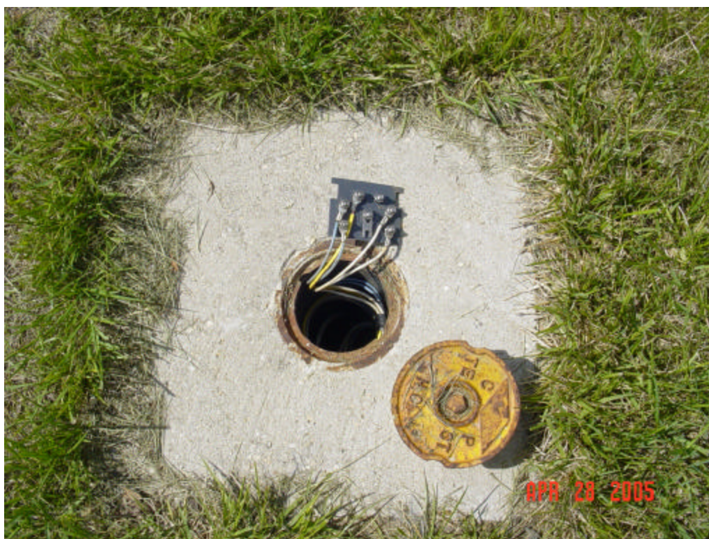
Figure 213 - Test Station 3811-9 close-up
