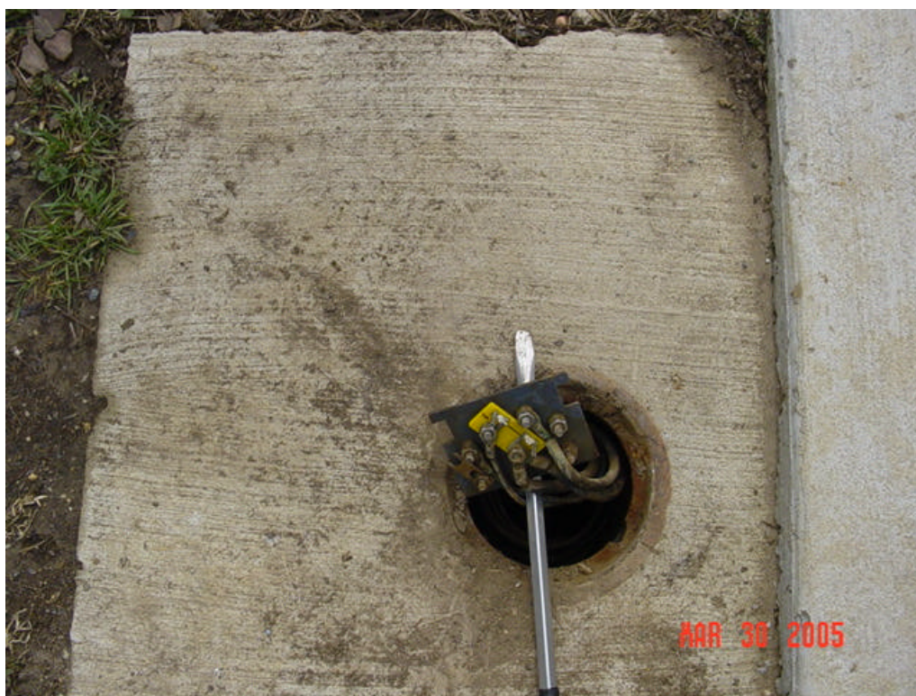
Figure 209 - Test Station 3811-7 close-up
