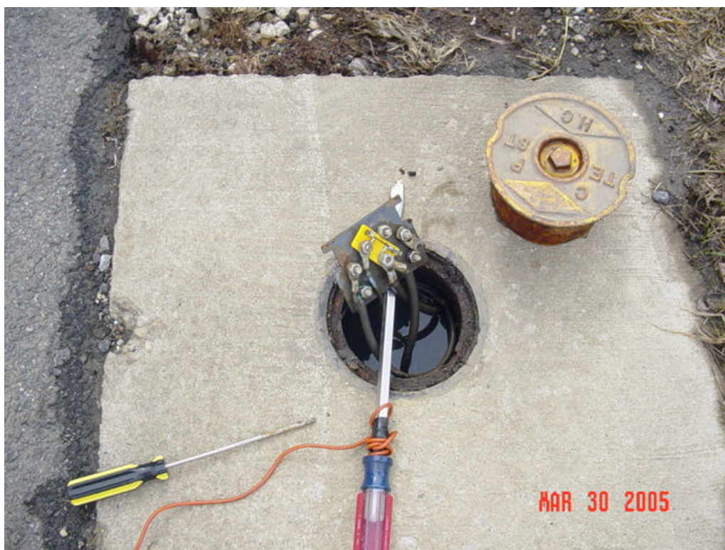
Figure 205 - Test Station 3811-5 close-up
