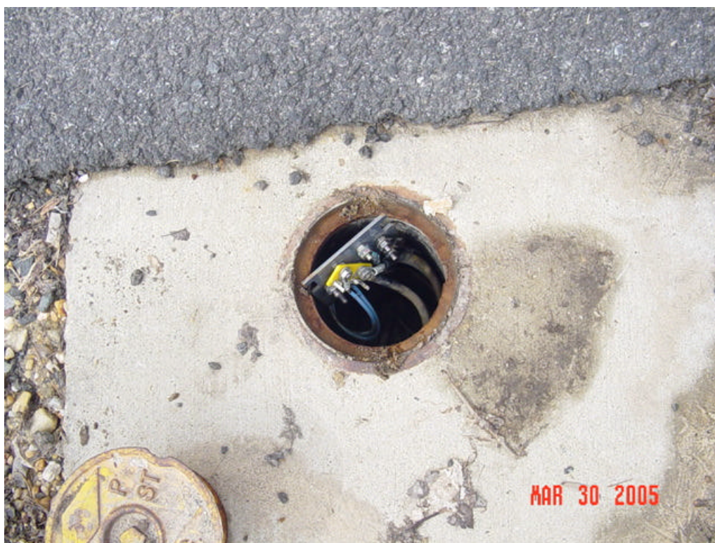
Figure 198 - Test Station 3811-1 close-up
