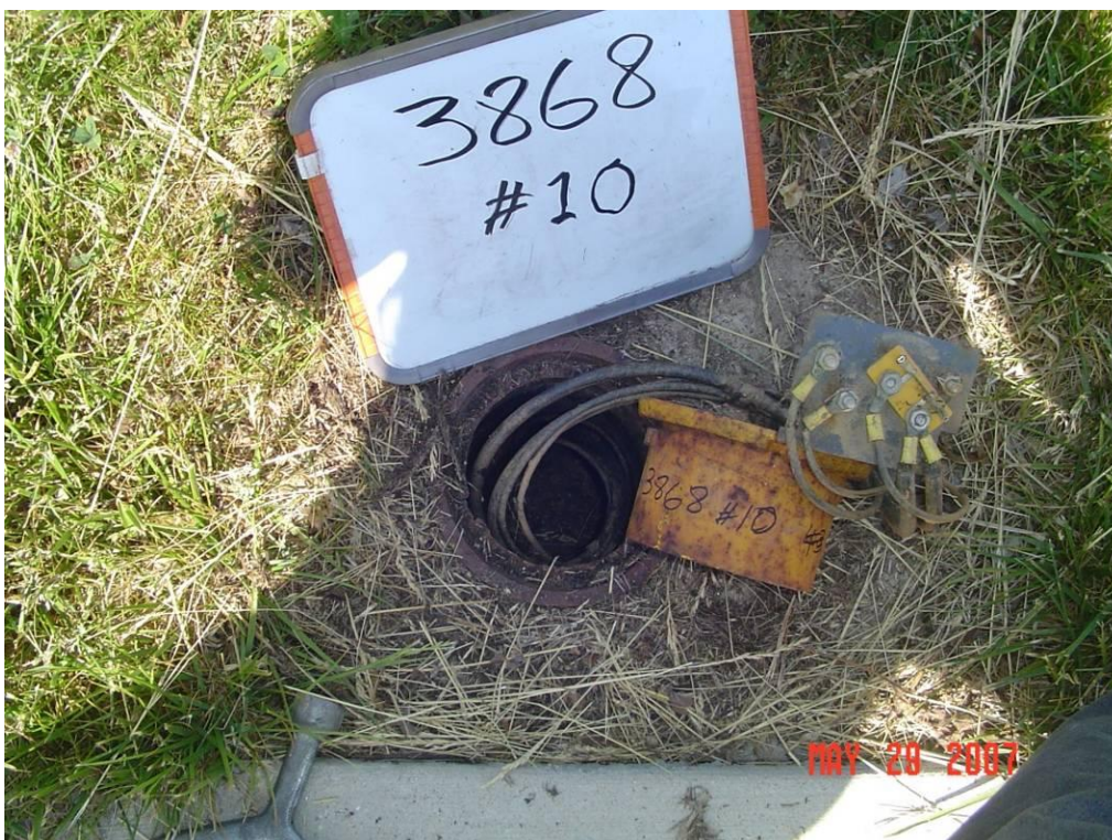
Figure 93 – Test Station 10 close up
