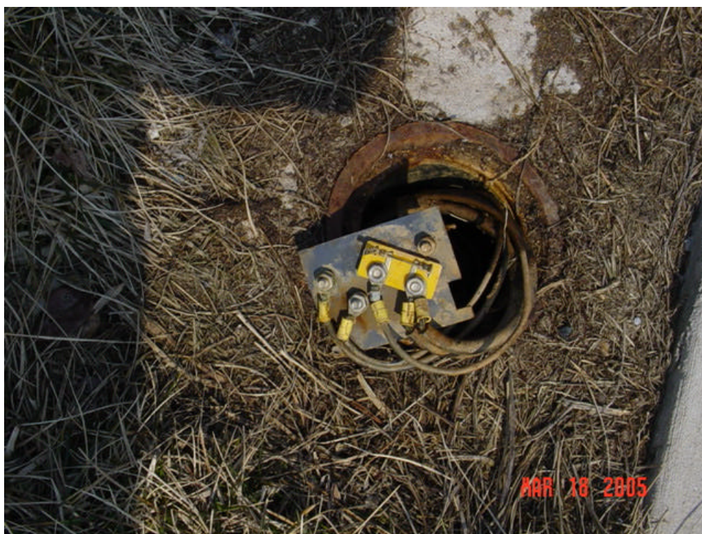
Figure 107 – Test Station 10 close up
