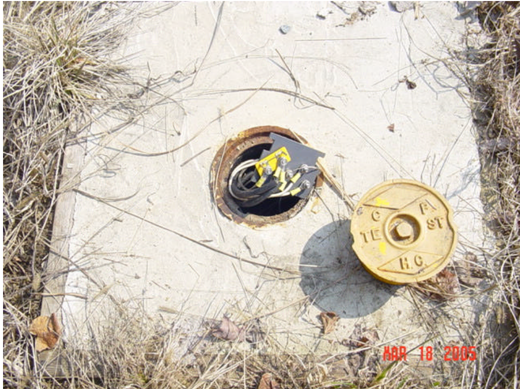
Figure 99 – Test Station 6 close up
