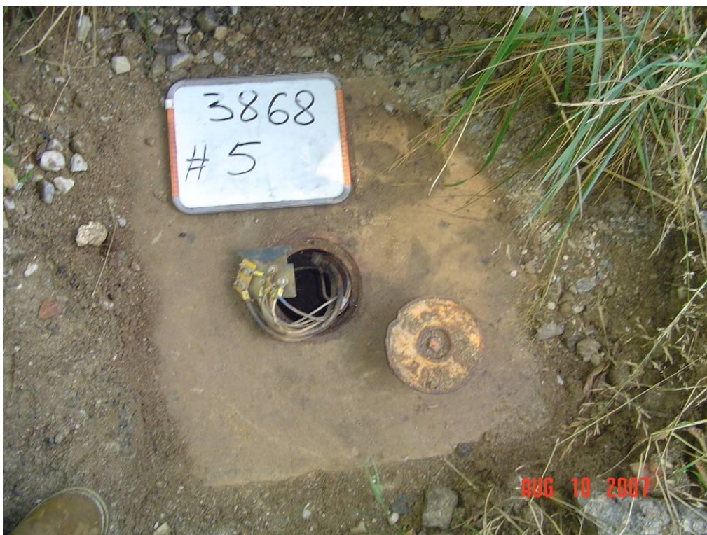
Figure 83 – Test Station 5 close up
