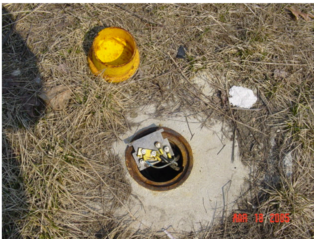
Figure 91 – Test Station 3A close up
