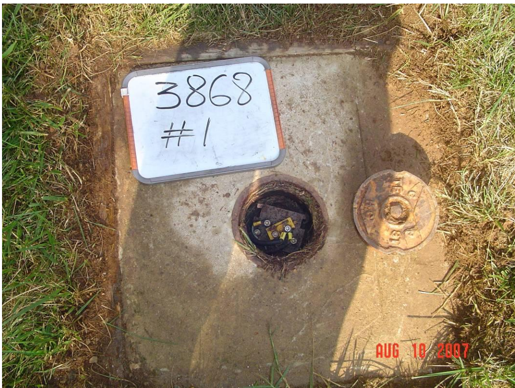
Figure 73 - Test Station 1 close up
