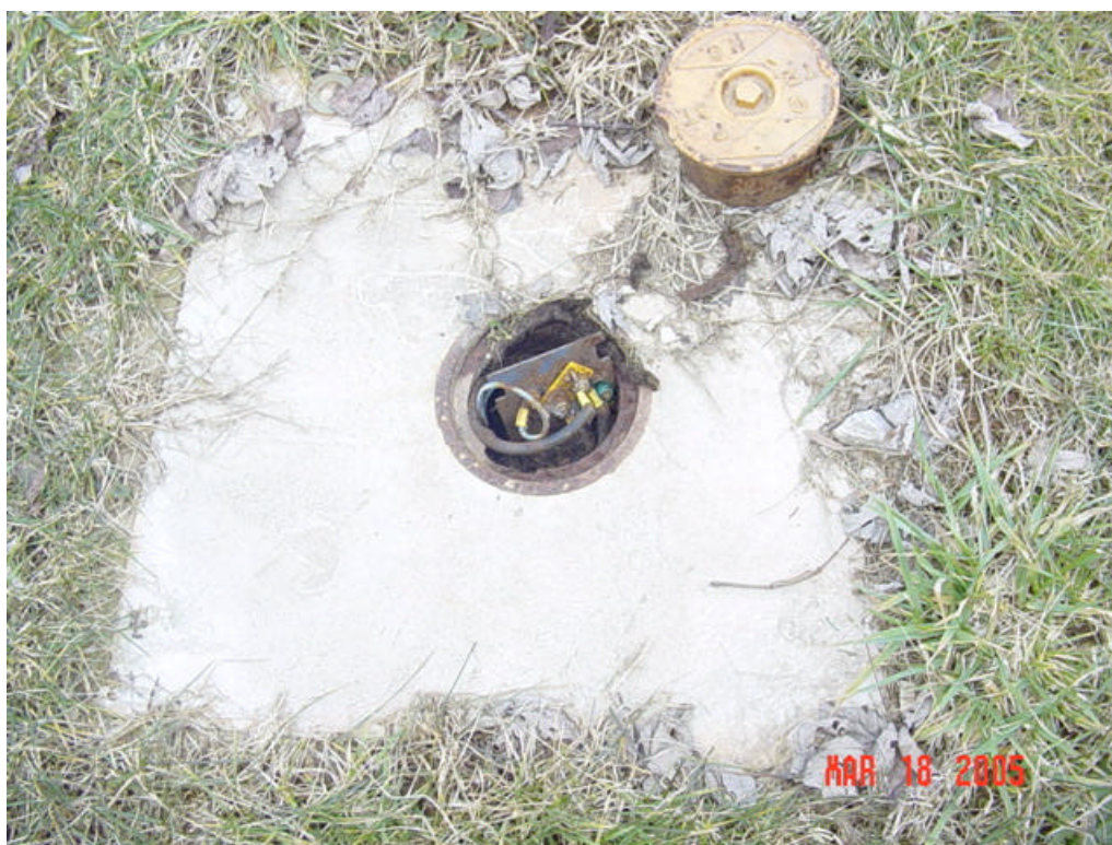
Figure 87 - Test Station 1 close up
