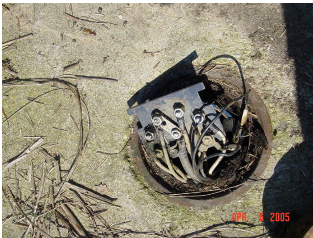
Figure 50 - Test Station 3725-3 close-up
