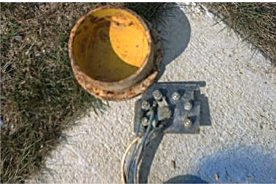
Figure 60 - Test station 175A, close-up
