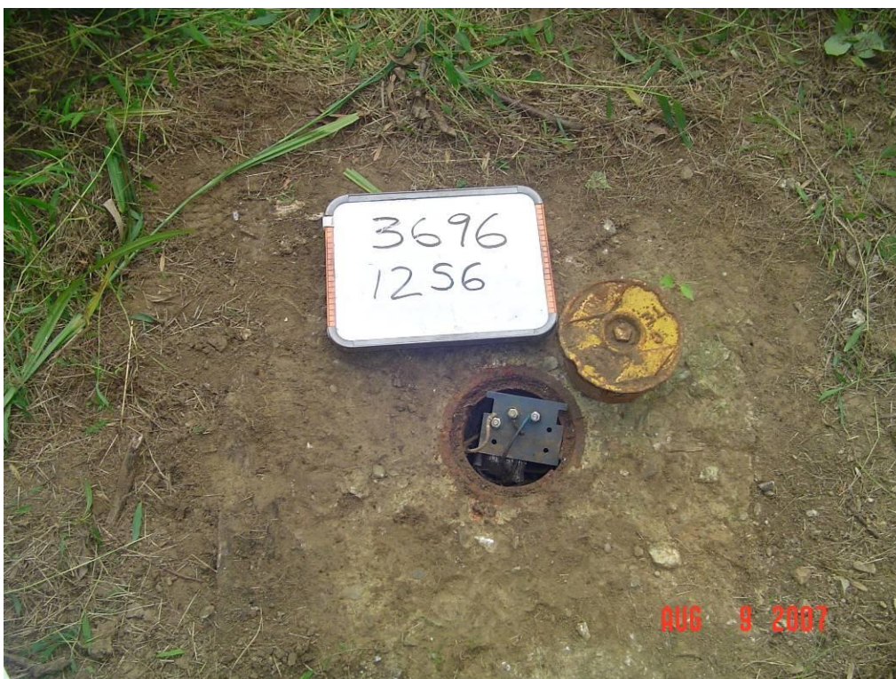
Figure 17 –Test Station 12GS6 close-up
