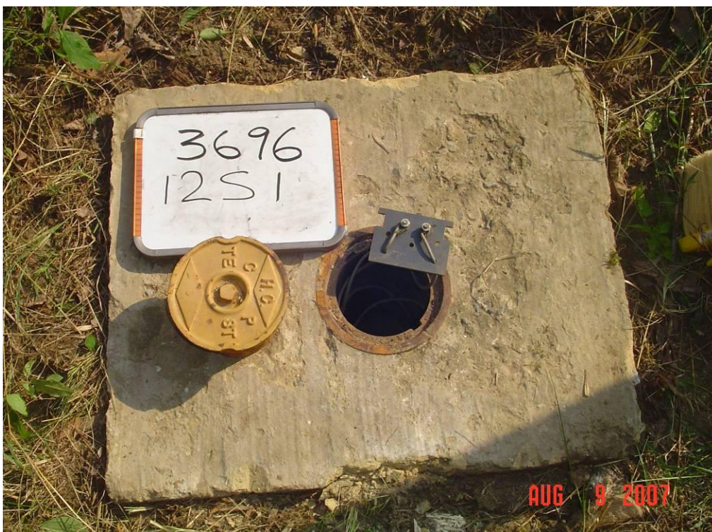
Figure 9 - Test Station 12GS1 close-up
