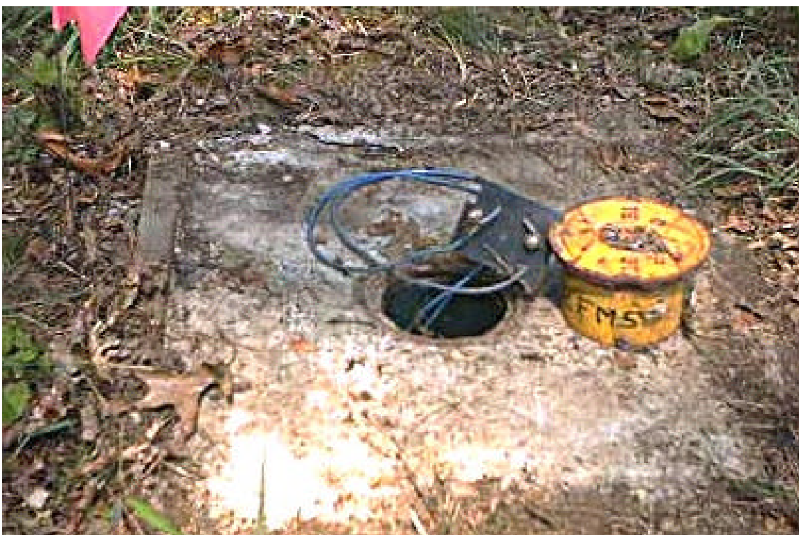
Figure 21 - Test station 12FM5, close-up
