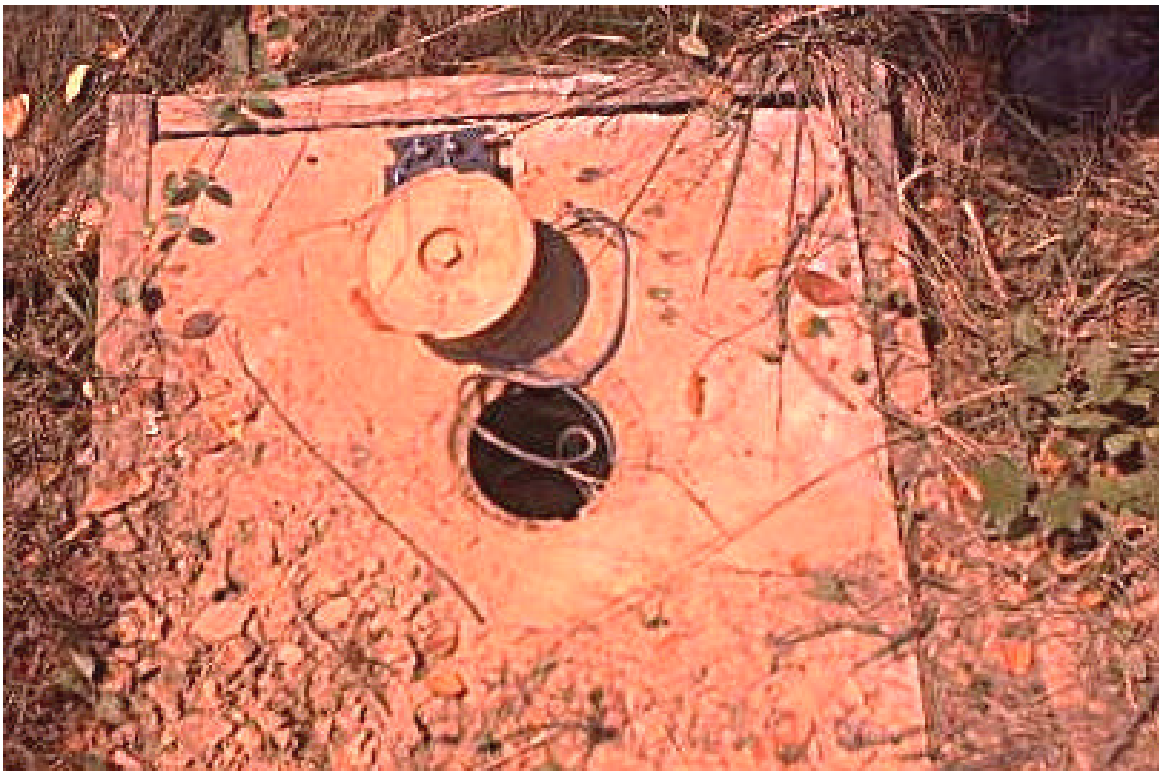
Figure 16 - Test station 12FM2, close-up
