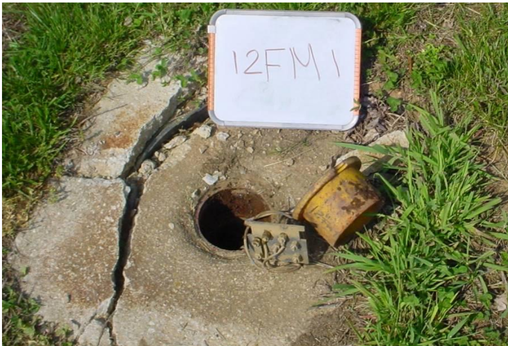
Figure 19 - Test Station 12FM1 close-up
