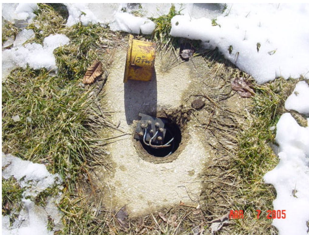
Figure 21 - Test Station 12FM1 close-up
