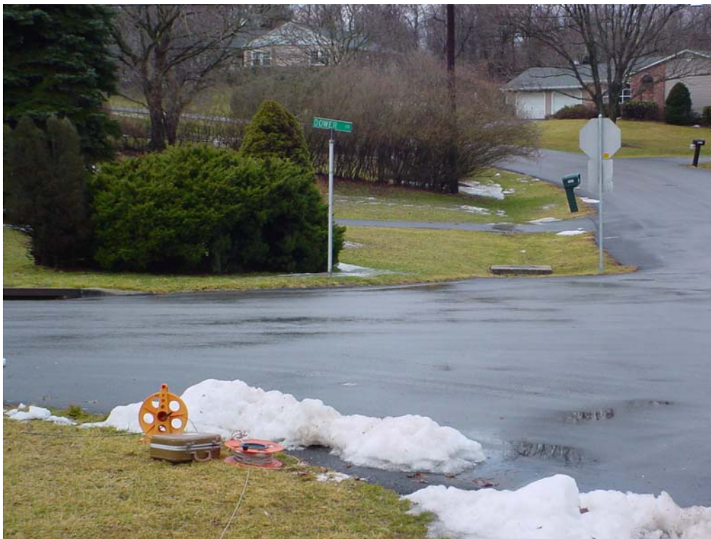
Figure 54 – Measuring stray currents near Dower Drive and East Leisure Court
