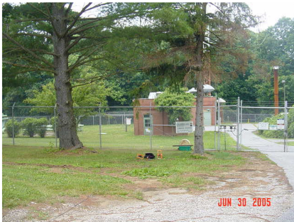
Figure 42 - Impressed Current Rectifier CMB1
