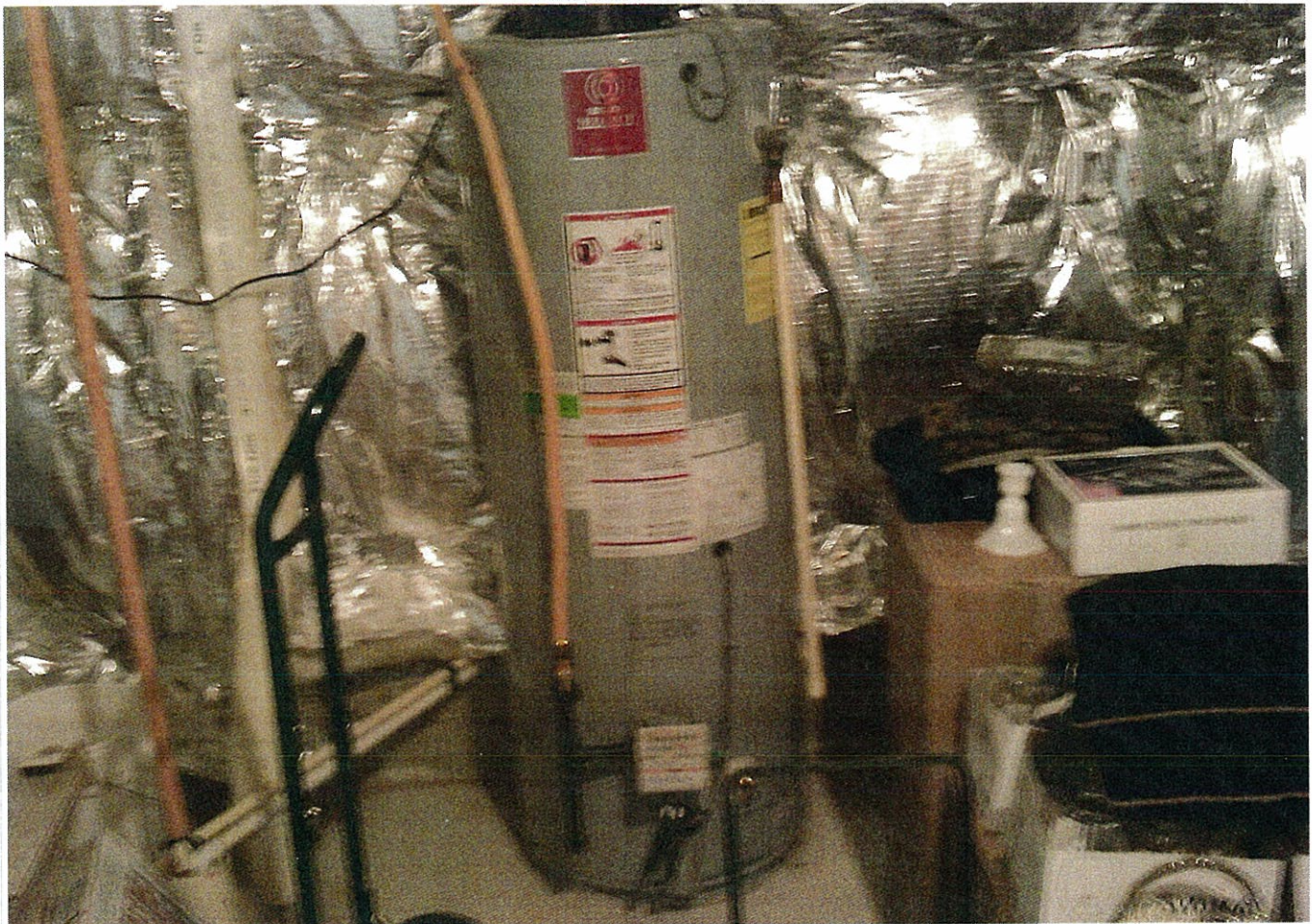
Hot water heater
