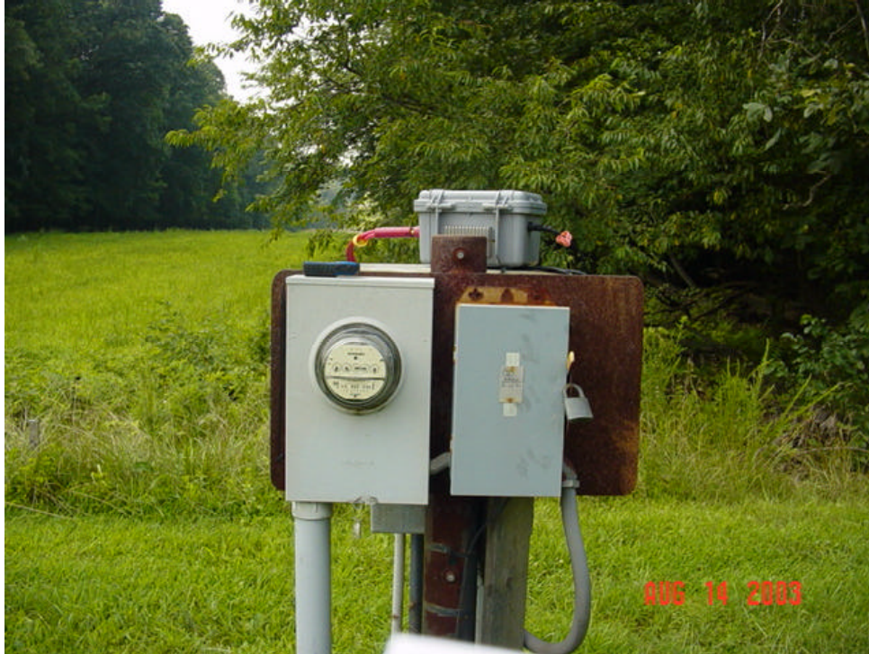
D 2 - Rectifier 190-1-1 located at the Marriotsville Landfill (N39E 18.2948', W76E 54.3356')
