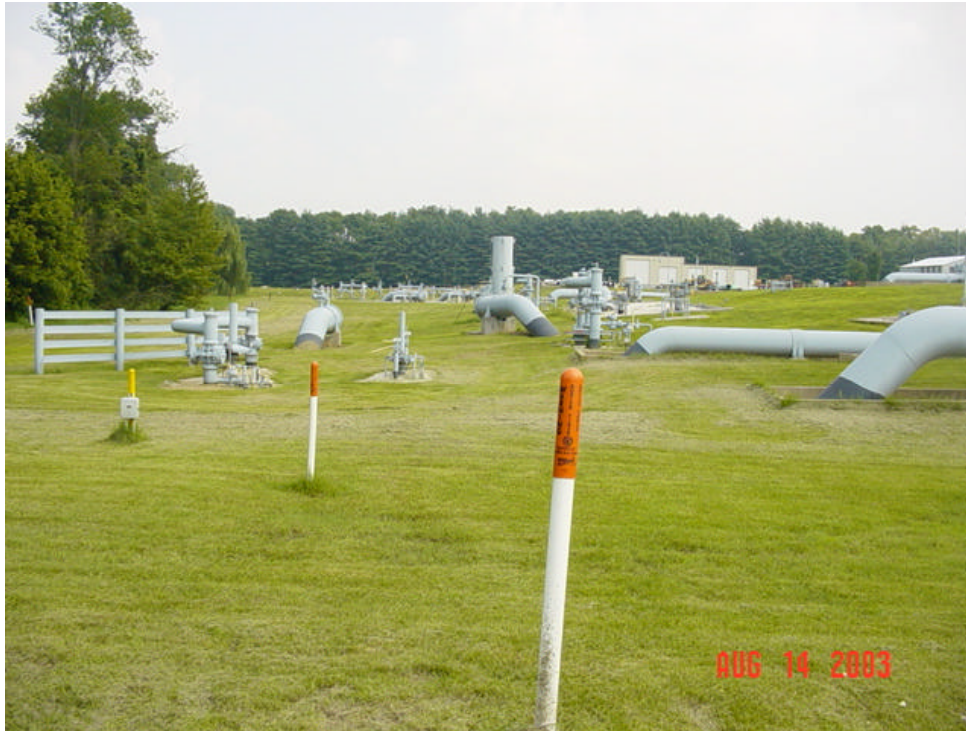
D 3 - Rectifier 190,190-0,190-0-1 Located at Carroll Mill Rd (N39E 15.9668', W76E 55.6829')
