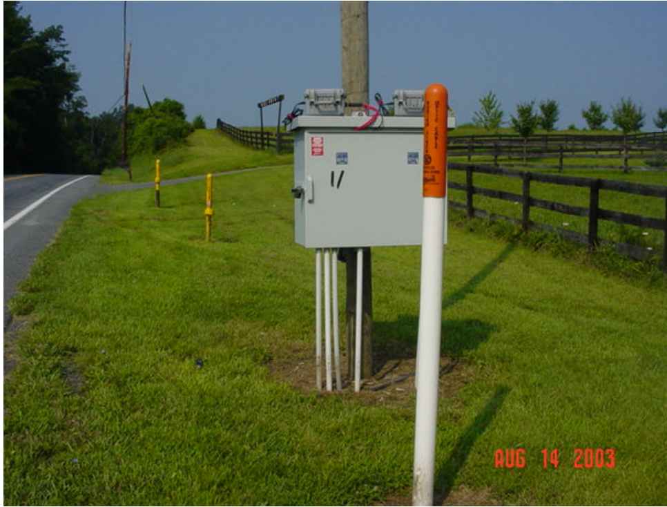
D 1 - Rectifier 190-1-3-A&B located on Hwy 99 (N39E19.0242', W76E53.7586')
