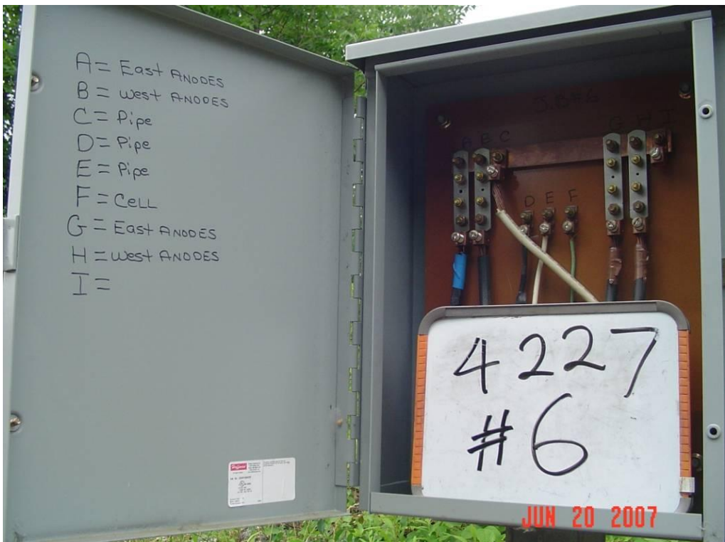
Figure 241 - Test Station 4227-6 close-up
