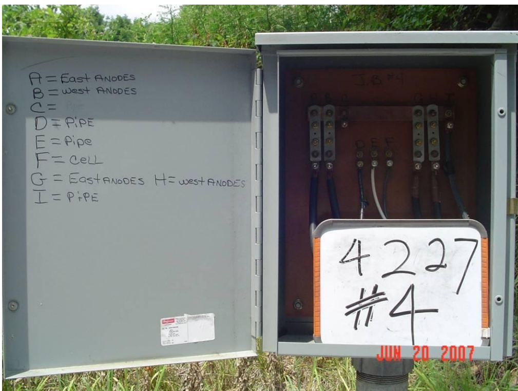
Figure 237 - Test Station 4227-4 close-up
