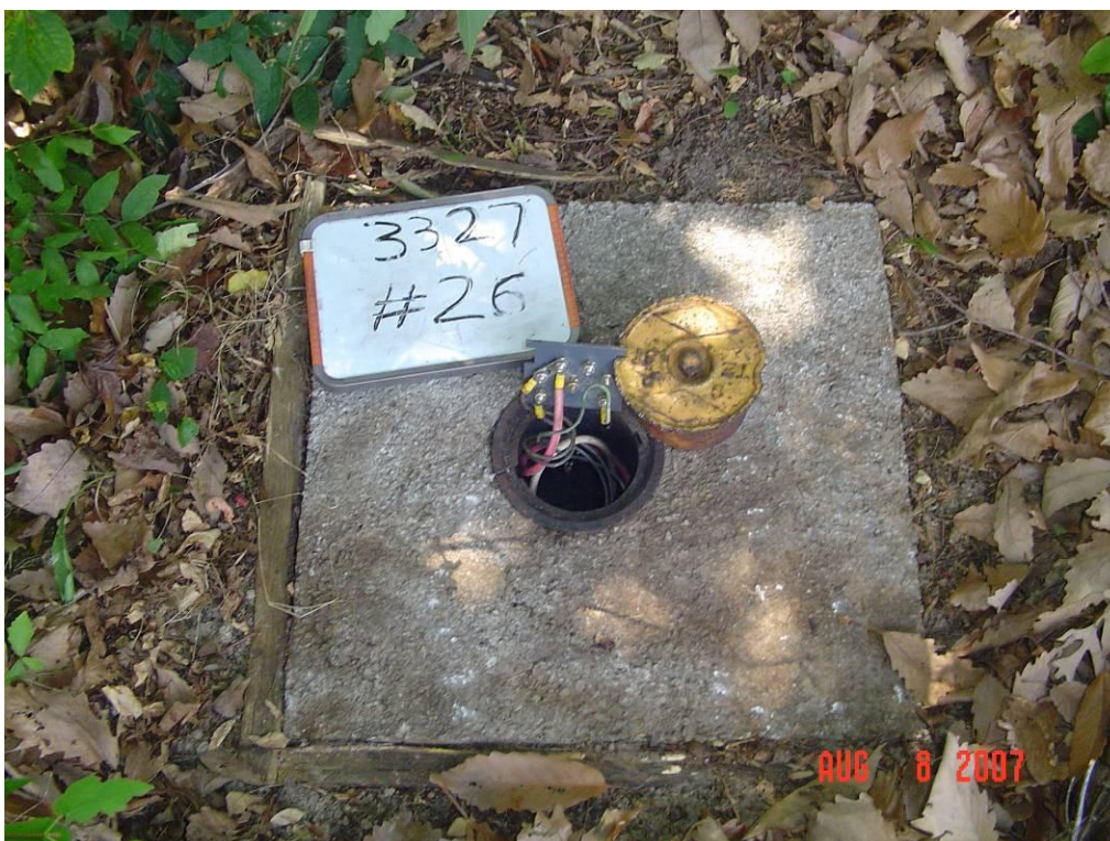
Figure 164 – Test Station 26 close up
