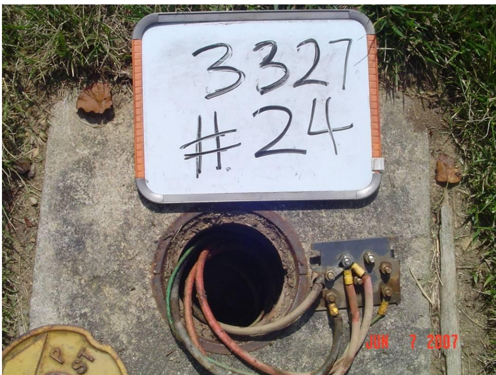
Figure 160 – Test Station 24 close up
