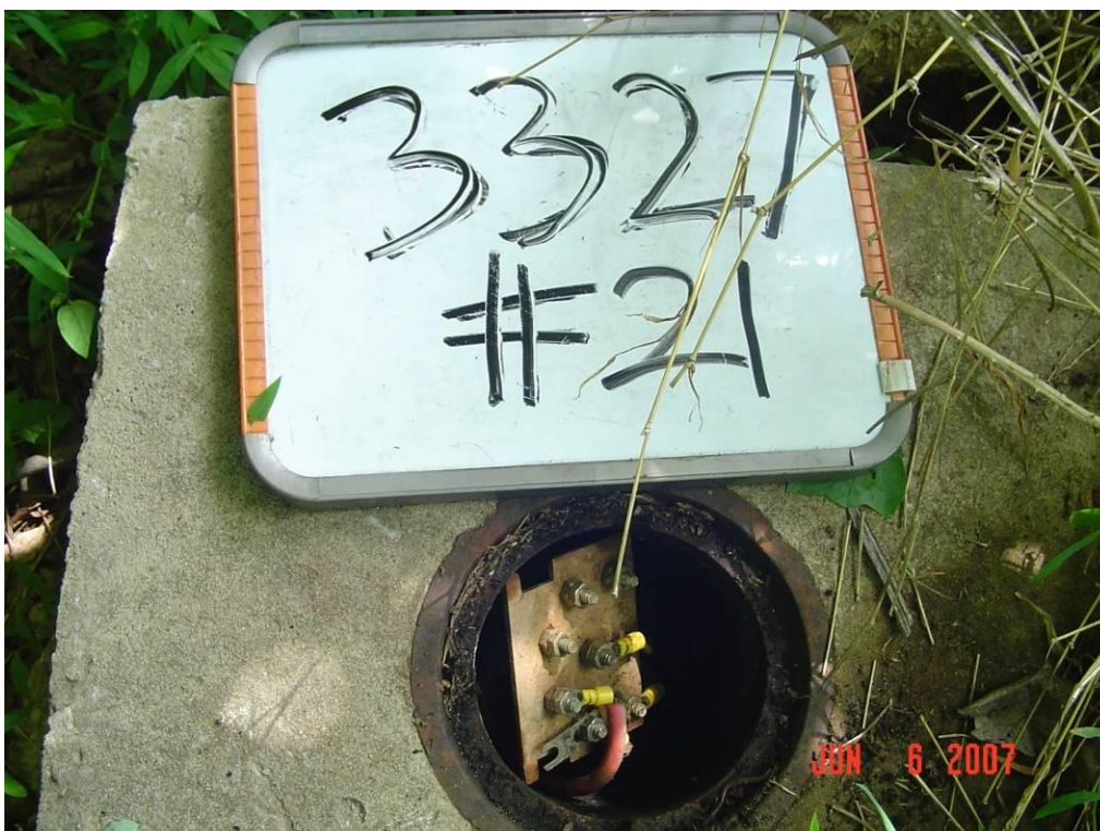
Figure 154 – Test Station 21 close up
