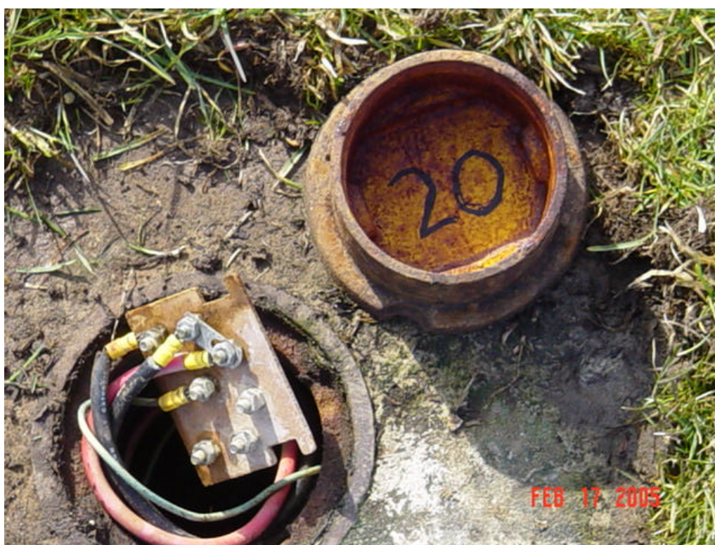
Figure 162 – Test Station 20 close up
