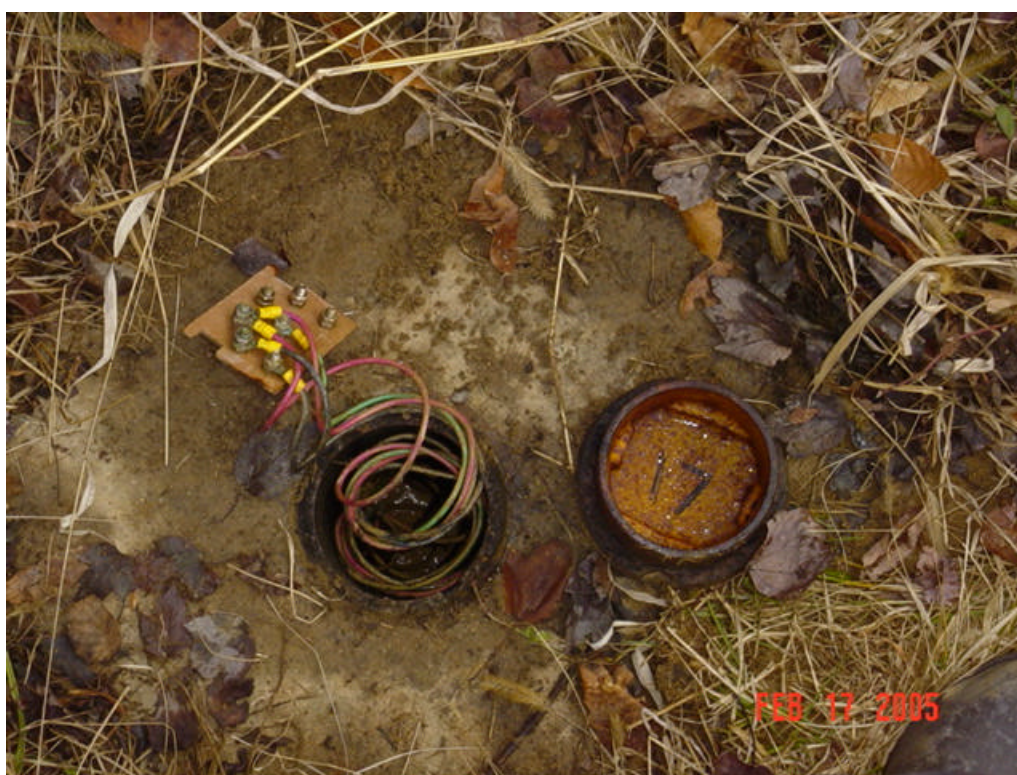
Figure 158 – Test Station 17 close up
