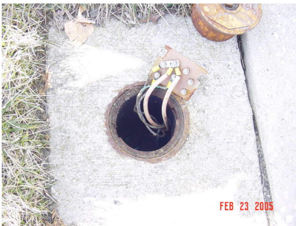
Figure 152 – Test Station 13 close up
